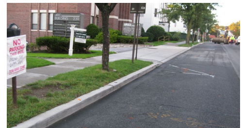
No parking on Broadway from 6pm - 7am due to gas construction. Other days had not parking 6am - 7pm
