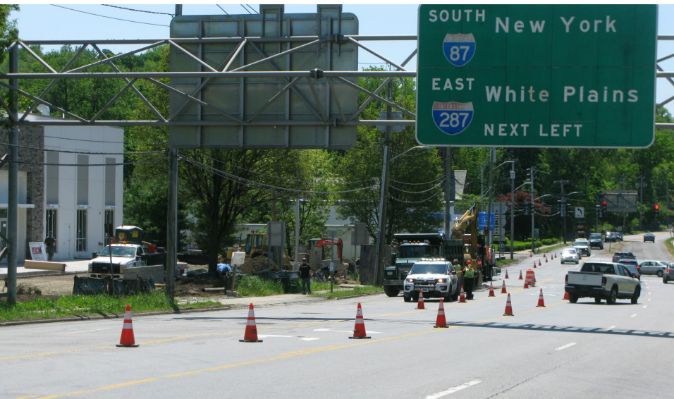
Above: People driving given clear path around construction zone at Honda dealership on 5/24/18.
