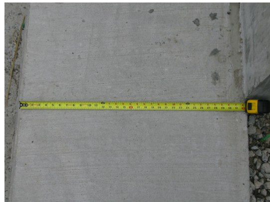
Beekman Ave Bridge's temporary sidewalk is just 32" wide at western end. ADA requires 36".
